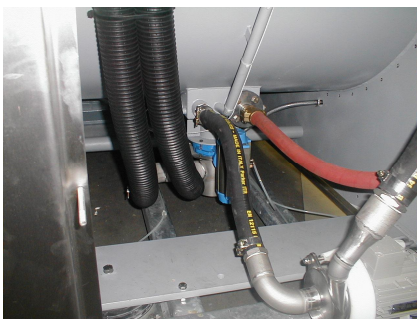
With discharge and recuperation pump
